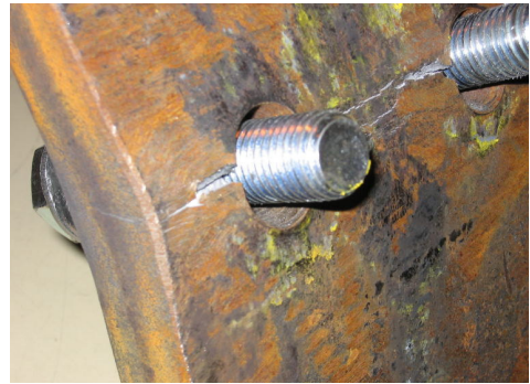
Figure 7: U device deformation with cracks.
