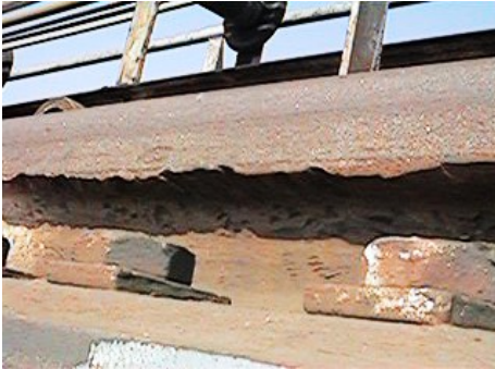
Figure 9: Erection defects – Case 3.
