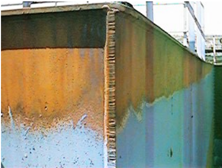
Figure 6: Fabrication defects – Case 3.
