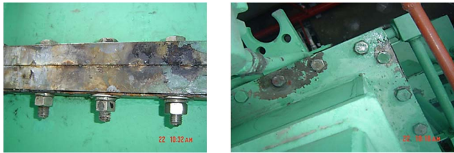
Fig. 15. (a) Paint loss due to overheating (zone 2: 386.9 °C) in the connection of flange-bolts (left). (b) Paint loss due to overheating (zone 1: 140.8 °C) in the connection of flange-bolts (right).
