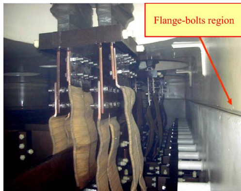
Fig. 2. Arrow shows the connection of flange-bolts inside the transformer.
