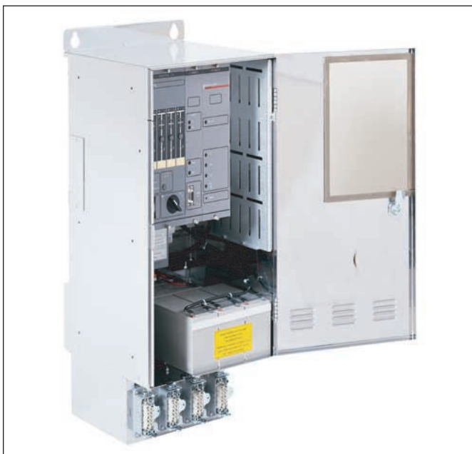
Figure 3. Integrated substation control unit for four feeders
