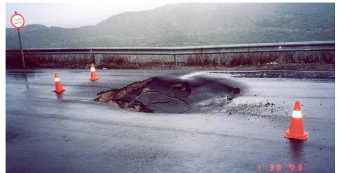
Fig. 8. Large pothole at the problematic section of the highway (from Dounias et al., 2006).
