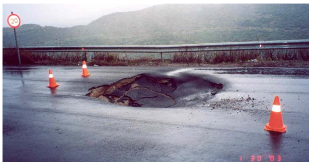
Figure 8: Large pothole at the problematic section of the highway (from Dounias et al., 2006).
