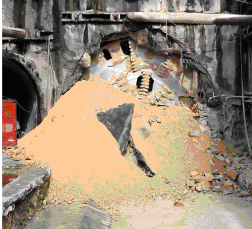
Figure 13: Final breakthrough of the TBM S-203 on the completion of the drive from Salgueiros to Trindade on Thursday 16 October 2003.
