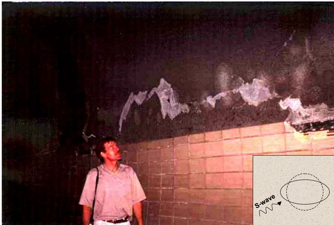
Longitudinal cracks from "ovalization" of Yuluh tunnel section, Chi-Chi 1999 earthquake (Schiff and Tang eds, 2000)
