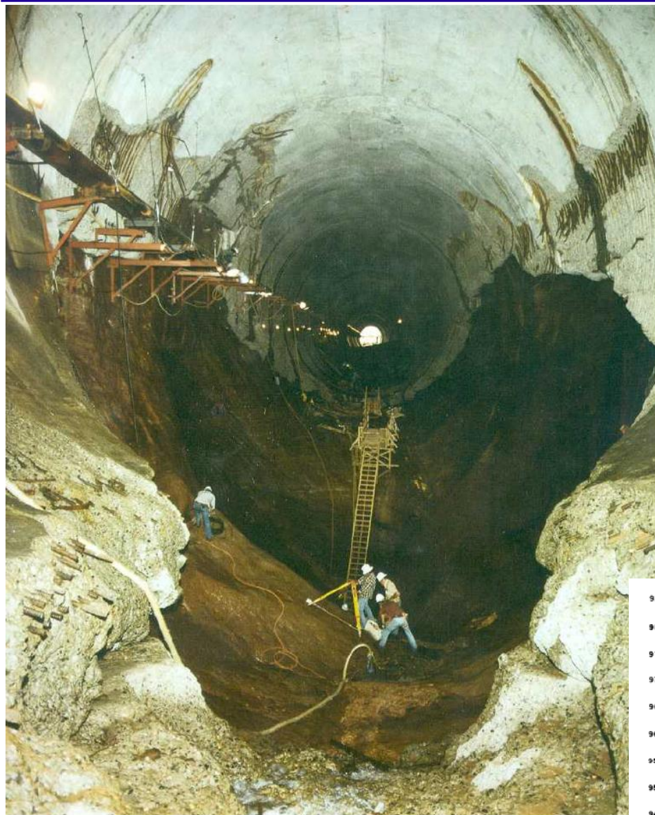
FRONTISPIECE.—Glen Canyon Dam. Left Spillway Tunnel Sept. 1983. The "big hole" in the spillway invert was 11 meters deep. Photo C557-400-690NA
