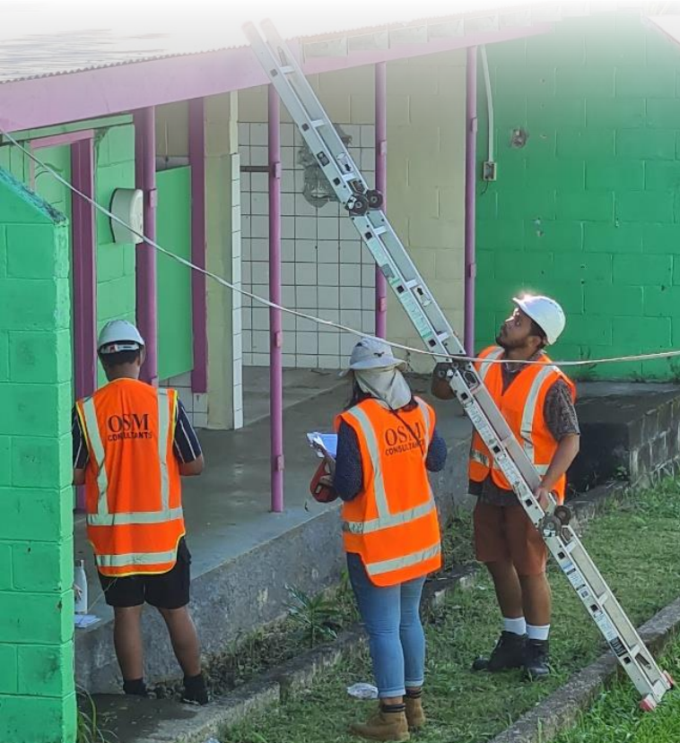
Building survey campaign in Samoa involved a local engineering firm and Ministry of Education and Training staff
